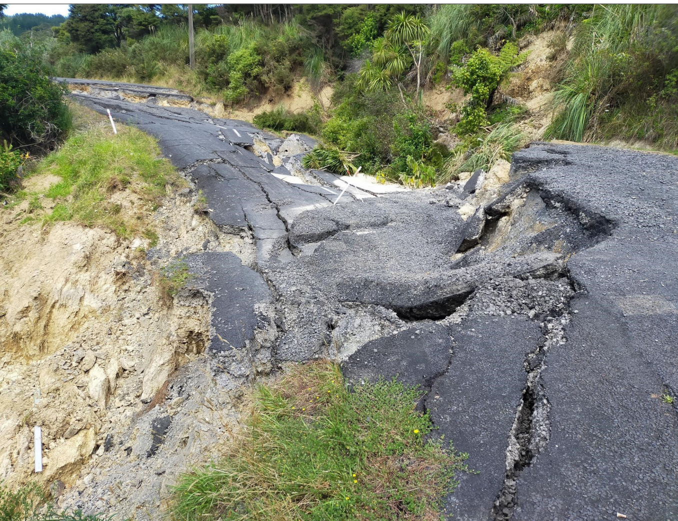
Damage to Port Waikato-Waikaretu Road as a result of Cyclone Gabrielle.
