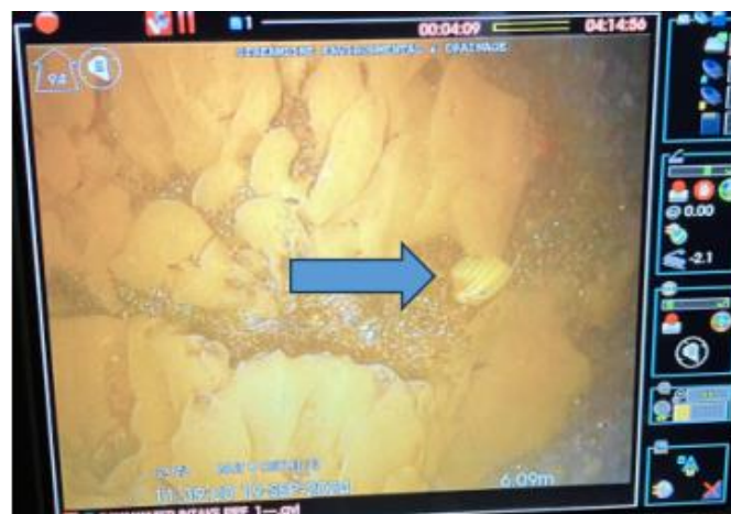
CCTV Footage of the internal pipe wall and clam
