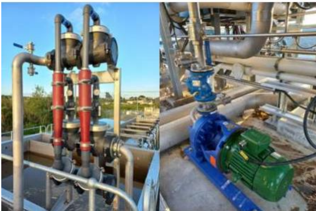
Te Kauwhata - Blower pipework
