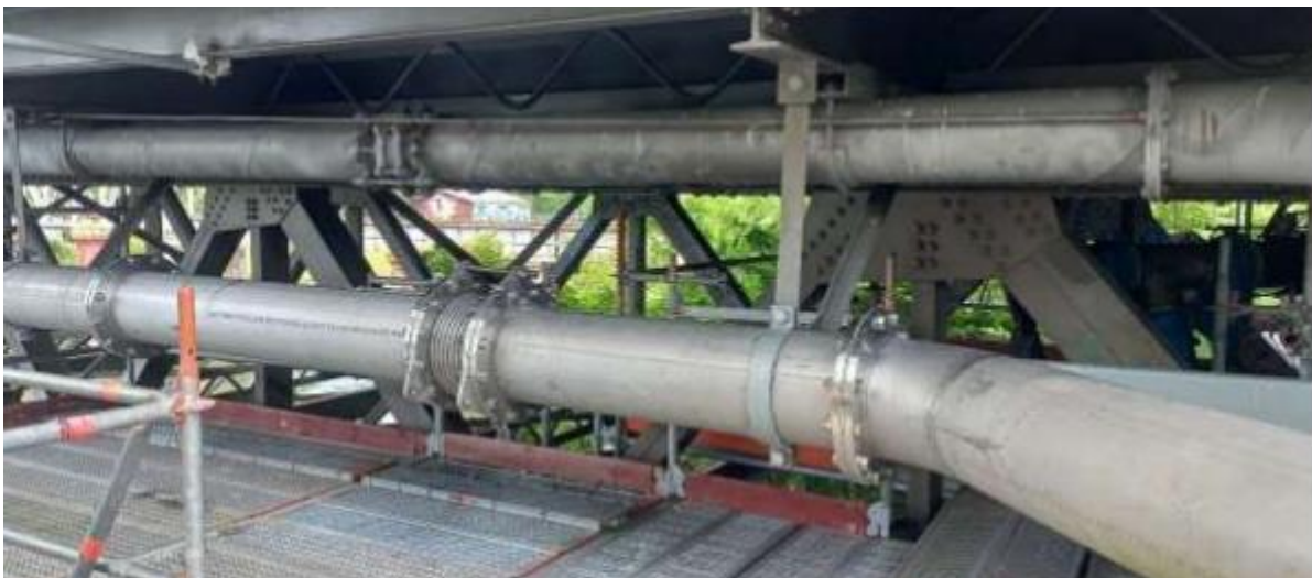
Ngaaruawaahioa pipeline - A new pipe spool installed under the Waikato River Bridge, diverting the Esplanade WWPS flow to the new sewer.
