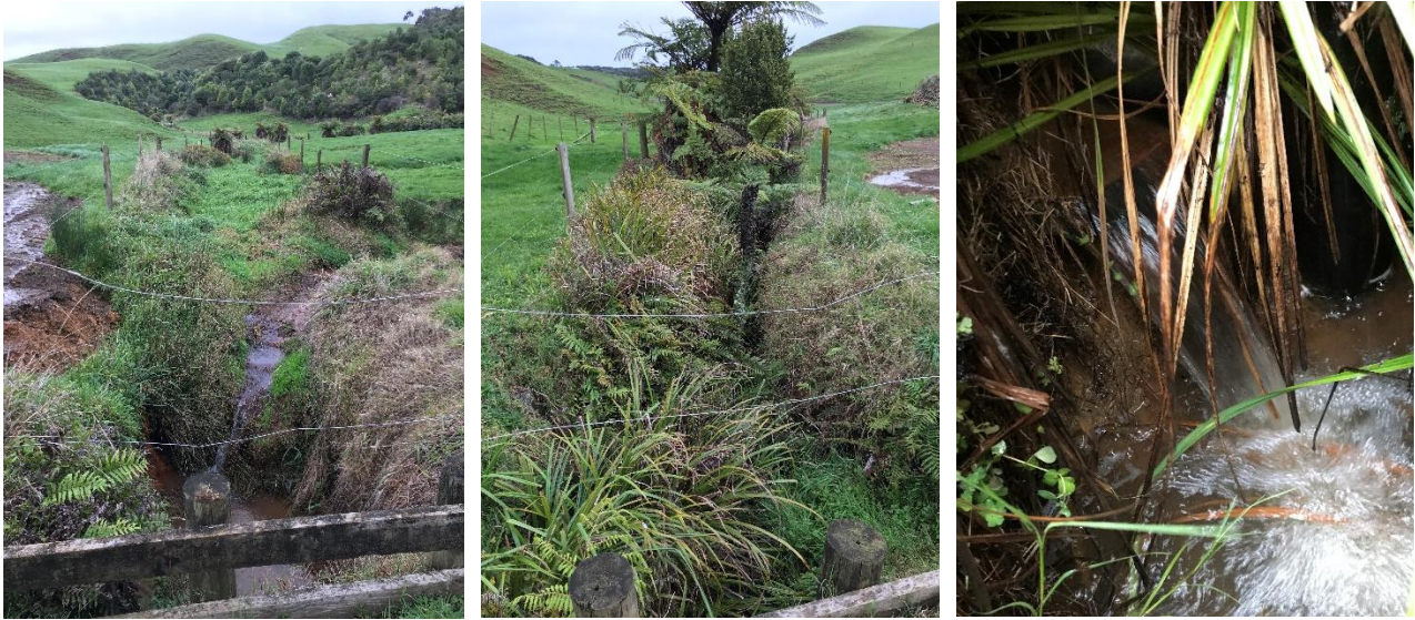
Figure 15. 15 Te Ahiawa Road tributary 3 - Photos from left: upstream of the bridge, downstream of bridge, perched culvert.
