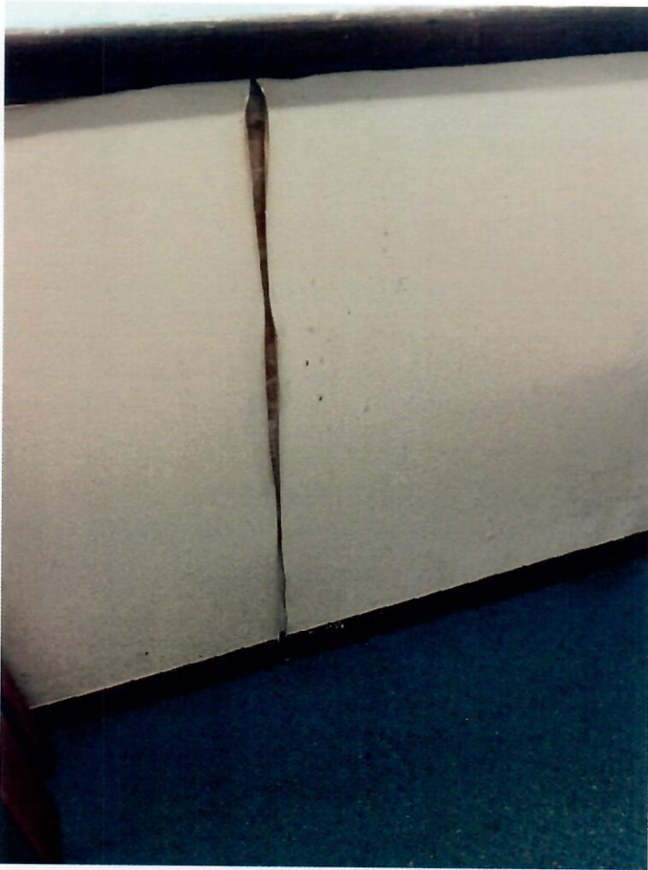
Photo showing wallpaper deterioration – January 2024
