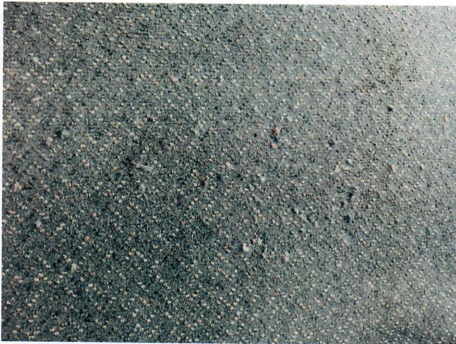
Photo of carpet showing wear and tear – January 2024
